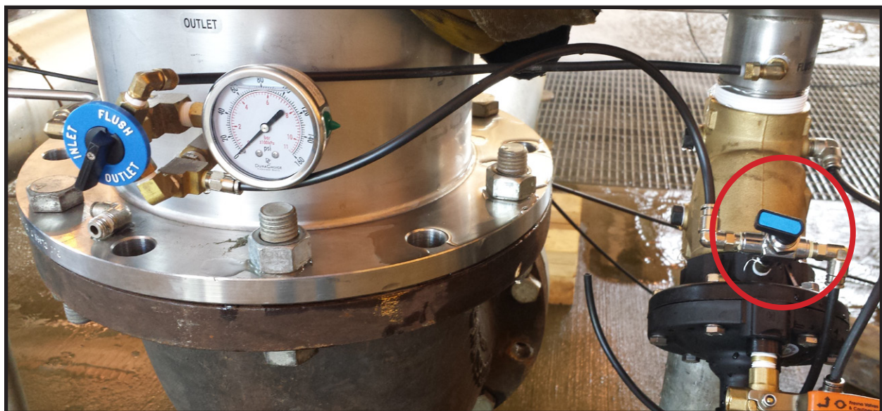
Photo of zero pressure in the FLUSH when the flush valve is open
