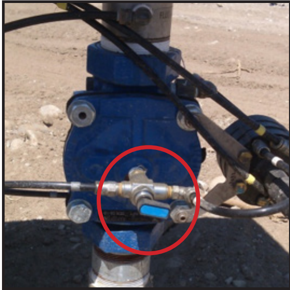
Flush valve in CLOSED position
