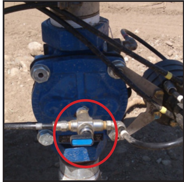
Flush valve in OPEN position
